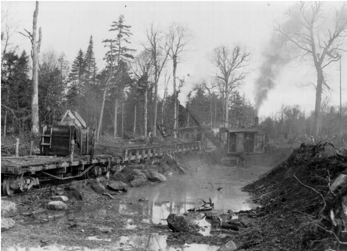
Eagle Lake & West Branch Railroad's Erie B2 steam shovel hard at work during construction of the railroad. This shovel now rests in a shallow pit near Nine Mile Bridge on the St. John River.
